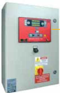
Control electric panel
